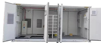
1075KW HH ESS
