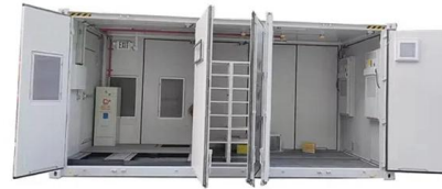
1075KW HH ESS
